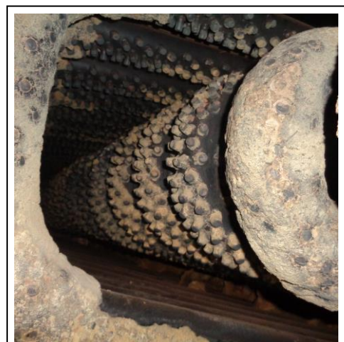
Photo 7: Ash slag over bed coil studs
