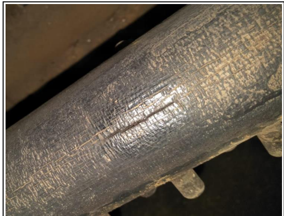
Photo 1: Cracks in the tube at top side
