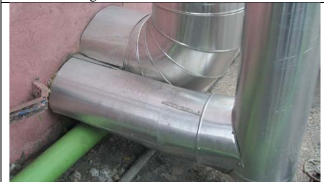
Photo 12: Steam piping to TG is seen buried in the TG building wall. This is a common mistake seen.
