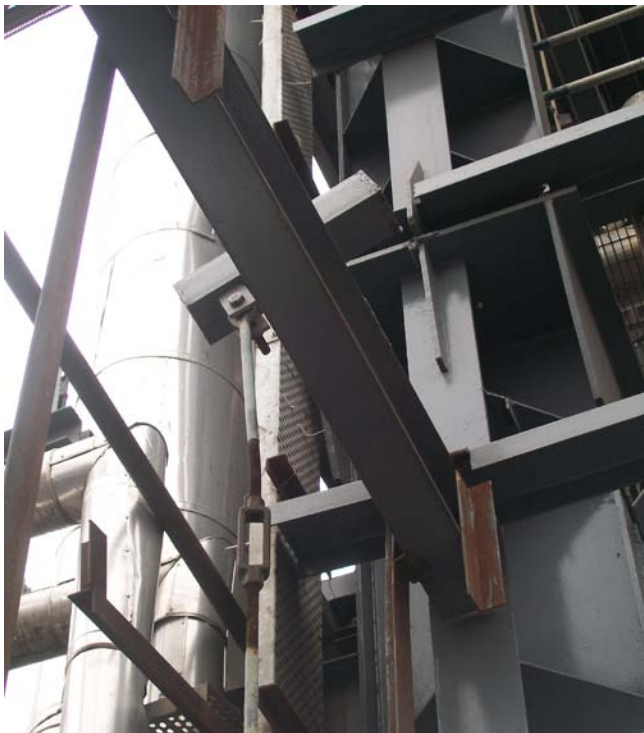
Photo 4: This is a mistake by a designer that a base support for hanger was not rigid enough. This is from another installation.
