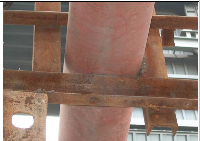
Photo 2: The steam piping from boiler no 2 to header is seen locked up. The insulation was removed to identify the temporary anchoring.
