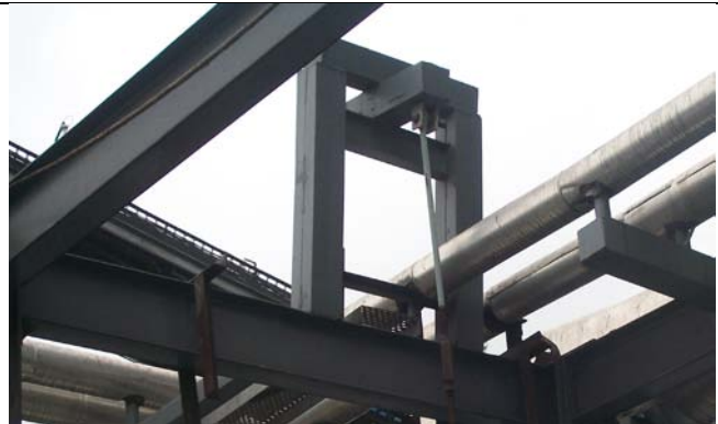
Photo 5: In the steam main steam piping, this is the status of the next support. The rigid hanger support base is not rigid enough.
