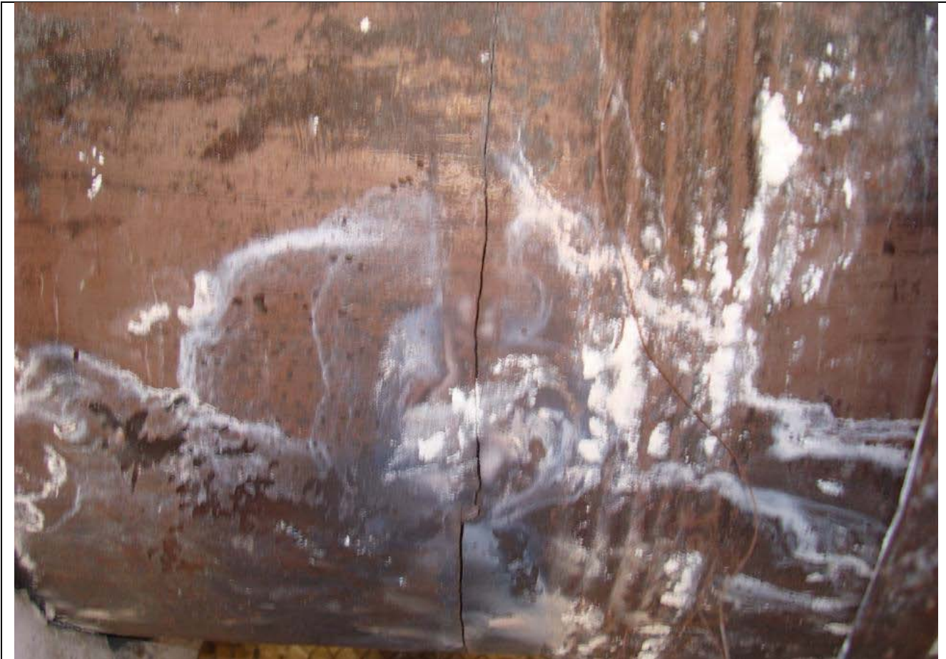
Photo 3: The header crack can be seen here very close to the weldment.
