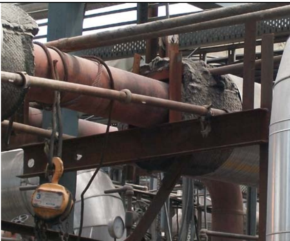
Photo 1: The steam piping from header to old TG is seen locked up. The insulation was removed to identify the temporary anchoring.
