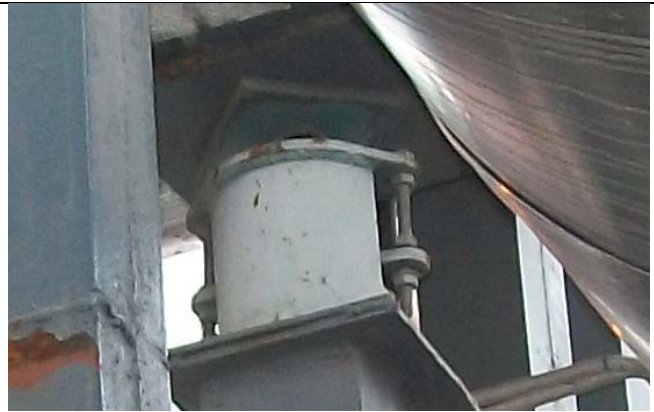
Photo 8: A spring support waiting to be loaded in the operating power plant.
