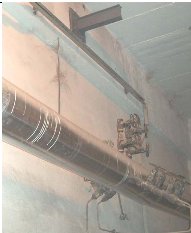
Photo 11: A rigid hanger in the boiler feed piping designed for 125 kg/cm 2 is seen fallen due to poor welding at support.
