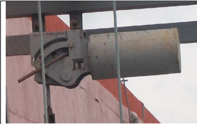
Photo 7: A constant load hanger is seen with an improvised lock at a recently commissioned installation.
