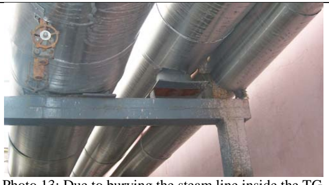
Photo 13: Due to burying the steam line inside the TG wall, the pipe support gets lifted off its sliding base.
